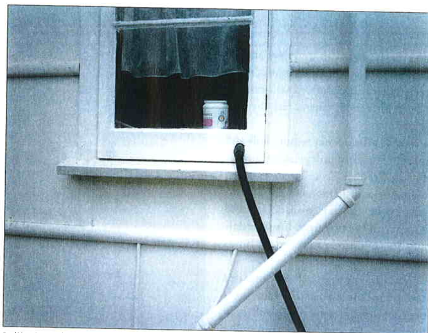
Drill a hole (with landlord's permission!) through a window frame to allow a hose from the laundry or bath to feed through to the garden.
